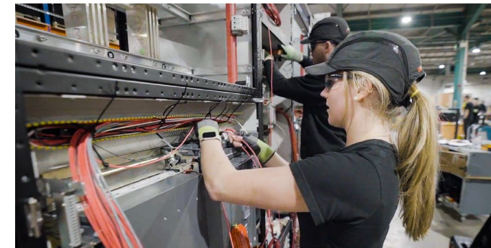
Switchgear assembly in Campsie, Northern Ireland
