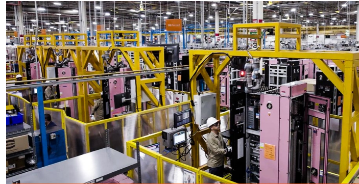
Power Distribution testing in Reynosa, Mexico
