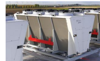
Data Center Cooling
