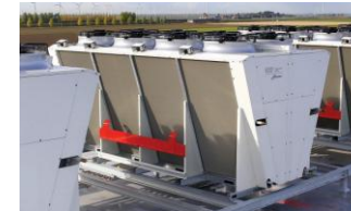
Data Center Cooling
