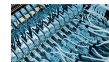
Commissioning Liquid –cooled DC
