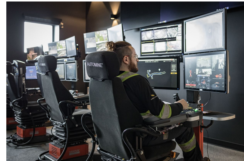
LaRonde Complex automation room
