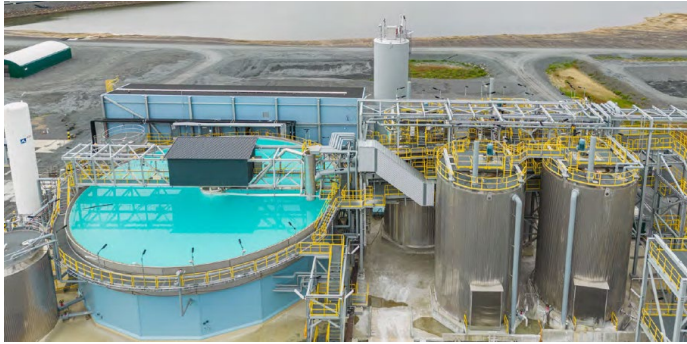
Kittila water treatment plant
