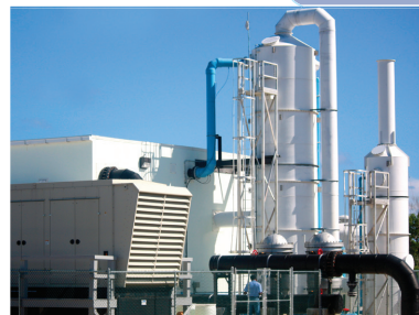
North Side Water Works plant Grand Cayman, Cayman Islands
