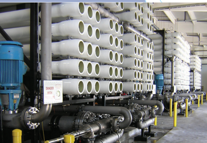
Membrane arrays at our Blue Hills plant Nassau, Bahamas
