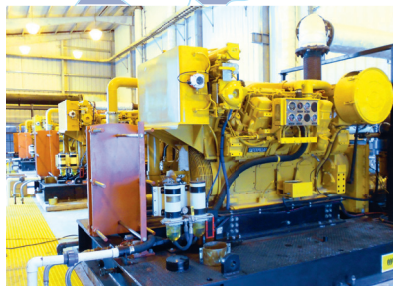
Diesel engines at the Blue Hills plant expansion Nassau, Bahamas
